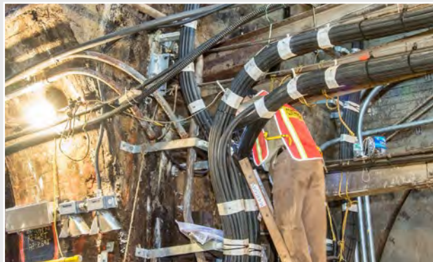
An L.K. Comstock electrician installs a serve to reduce stress on the cables when routed off of the messenger bundles. This was a routine practice on this project to safeguard a lasting installation, projected to remain functional for up to 60 years.
