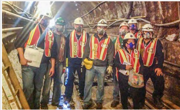
Because of the urgent nature of the project and the resulting tight schedule, L.K. Comstock performed site surveys while the demolition was taking place in the tunnel. Team members were trained and fitted for respirators to ensure a safe work environment in the tunnel.
