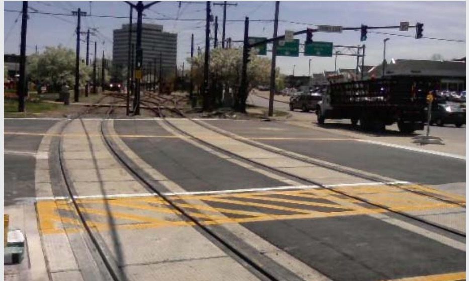
Crews reconstructed the crossing on Farnsleigh Road, the first of four double-track crossings reconstructed on the Greater Cleveland Regional Transit Authority light rail system.
