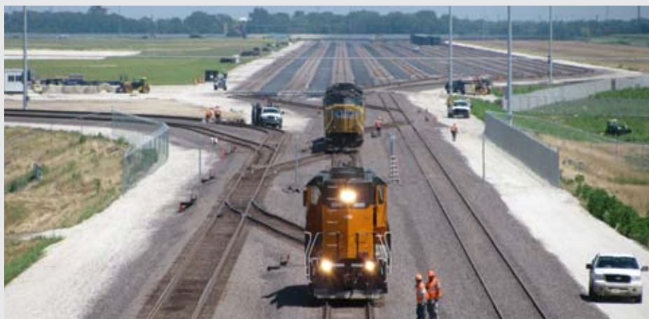
RailWorks' work-train locomotive and a Union Pacific locomotive headed south from the nearly completed CenterPoint Intermodal Facility in Joliet, Ill.
