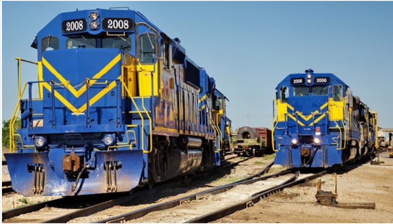
After earning a maintenance contract with Fort Worth & Western Railroad, RailWorks was awarded a capital contract to update Hodge Yard, pictured here. RailWorks is changing out six switches and additional panelized track in the yard, located in Fort Worth, TX.
