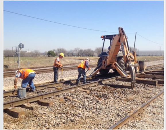
A RailWorks Track Systems crew changes out ties in Hodge Yard as part of ongoing maintenance.
