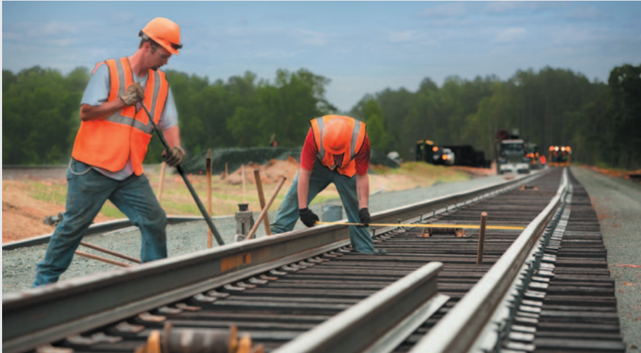
RailWorks Track Systems was not deterred from its job of constructing new track for the Western Wake Freeway project in Apex, N.C., during April, even after a tornado caused extensive damage in the area.
