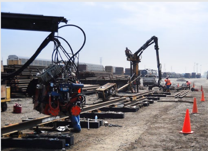
RailWorks Track Services set up a flash-butt welding process in CN's Kirk Yard to efficiently weld rail strings for new rail track construction.
