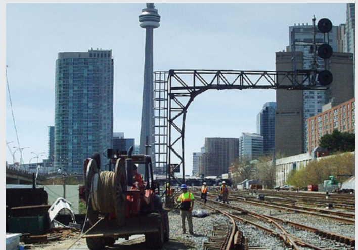
PNR RailWorks won a five-year contract to perform track and signal maintenance for GO Transit.
