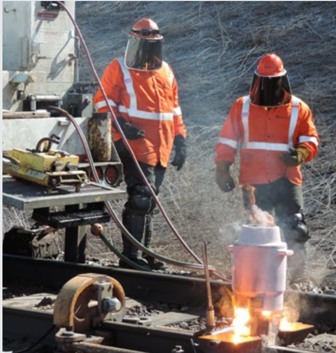
Welding crew members James Love and Brandon Robertson de-stress a portion of the Burlington Northern Santa Fe (BNSF) River Line in Lynxville, WI. All the Maintenance of Way crews perform thermite welds – by far the majority of the group’s work – with a handful of combo crews also performing electrical welds.
