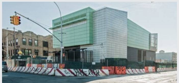
NY Transit crews have performed the civil and electrical work for the new, two-story relay room, which will replace a smaller, outdated relay room dating back to the 1950s. The new structure features the latest communications, fiber optic network, security controls, inergen fire protection and associated HVAC equipment systems, as well as new communications-based train control (CBTC) signal system technology.
