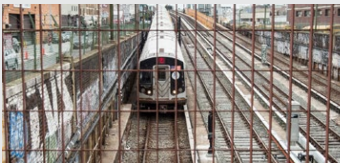
Three of the four Church Avenue mainline tracks have been reconstructed and placed into service. The remaining track will be completed in November. Crews reconstructed 216 insulated joint locations and 16 special portions of trackwork, with work being completed on select tracks during weekend outages while live train operations continued on the others.
