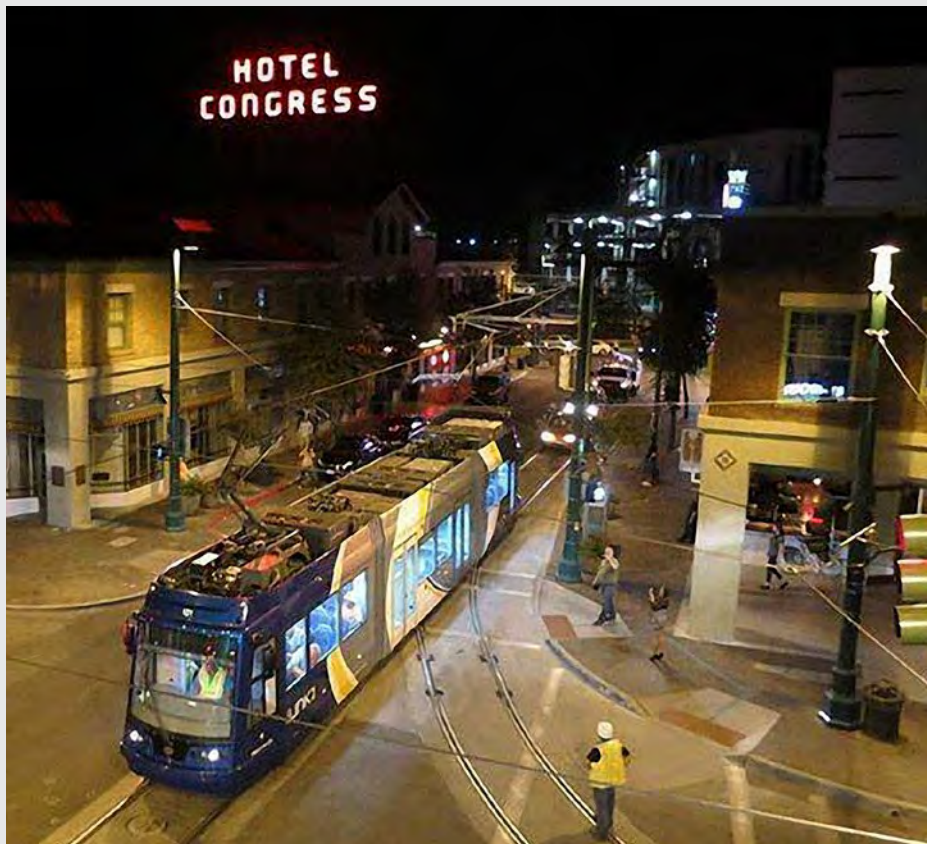
RailWorks has just wrapped up its work on the Tucson Modern Streetcar project, Sun Link. Extensive daytime and nighttime testing in October includes performing live-wire tests of the overhead catenary system, occurring here on East Congress Street at North 5th Avenue.
