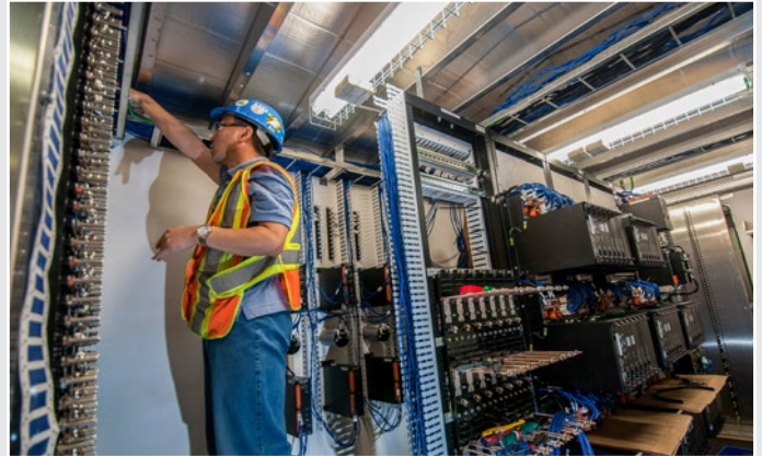
PNR RailWorks Signals & Communications Division constructed, wired and tested all 37 bungalows for the Georgetown South project in its Guelph, ON, wiring shop.
