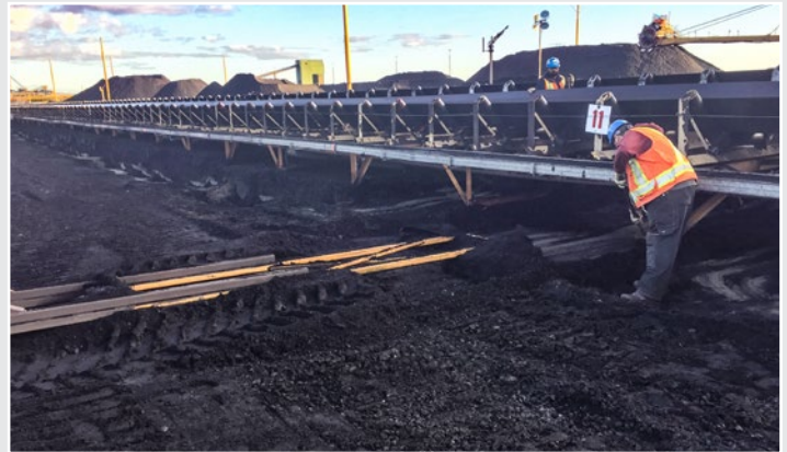
At Westshore Terminals, PNR RailWorks Trackman Inderjit Manhas removes coal from under conveyors to prepare grade for a contractor to pave.
