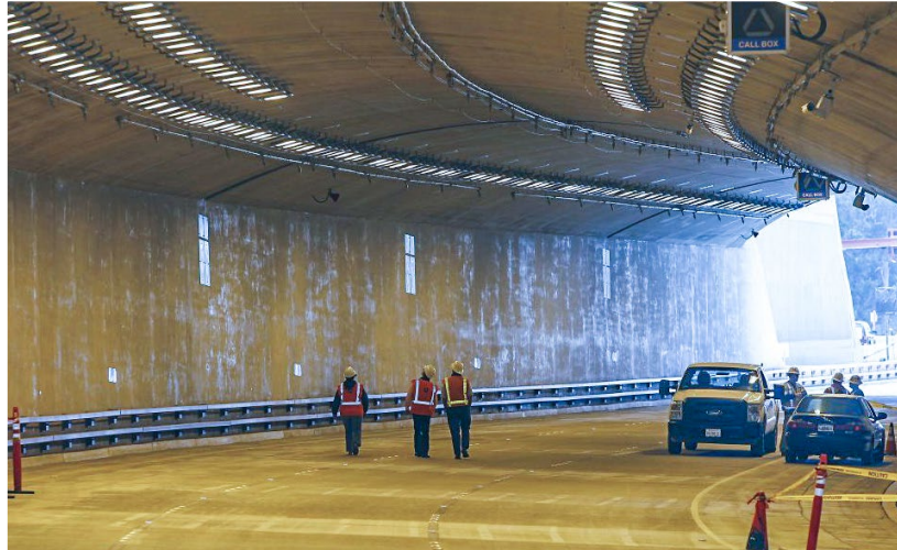
In San Francisco, HSQ Technology Project Manager Peter Waenink, second from far right, discusses emergency call boxes and associated wiring inside one of two new northbound Presidio Parkway tunnels. The Presidio Parkway project replaced an aging roadway with four tunnels, highways and viaducts in and near the historical Presidio national park district.
