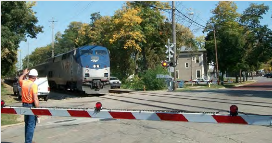
RailWorks Signals & Communications is installing positive train control (PTC) in Indiana and Michigan along Amtrak's Chicago-Detroit rail corridor. When the project is completed in late-2010, this corridor will be the first US rail line to be updated with new PTC technology.
