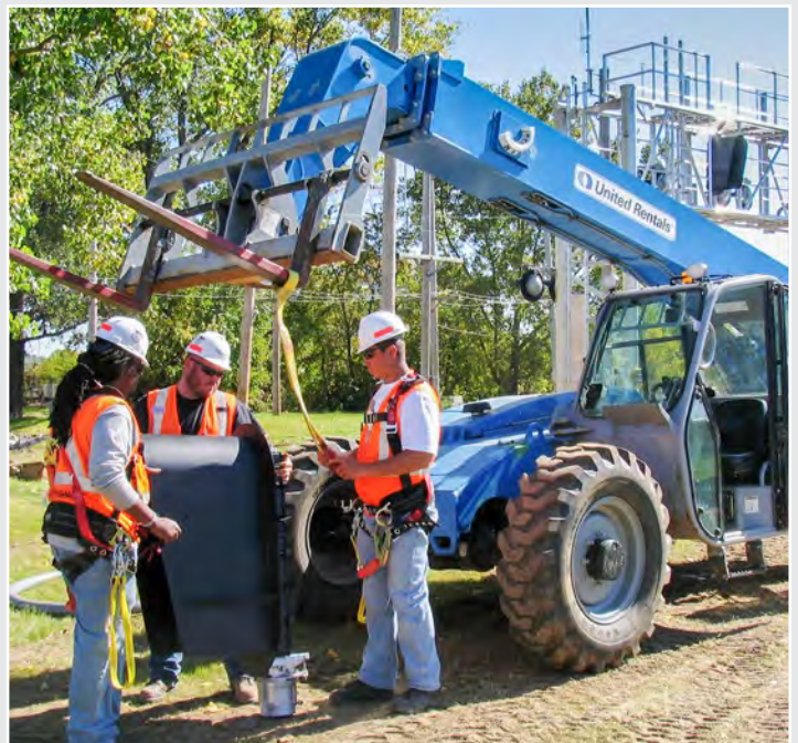
Equipment Operator Tony Golston , Foreman Brian Beard and Laborer Chris Koontz prepare a signal head to install on the new cantilever bridge. All three are new to RailWorks and the S&C division. This was the first S&C project for Tony and Chris, who were hired at an S&C job fair in Kansas City in mid-September.
