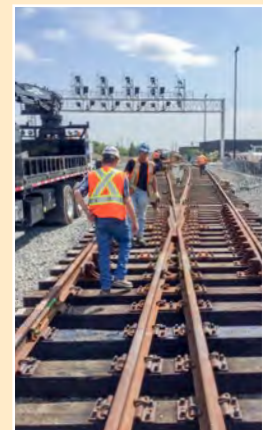
About 80 percent of track work for the Georgetown South project has been performed by PNR RailWorks' Eastern Division.
