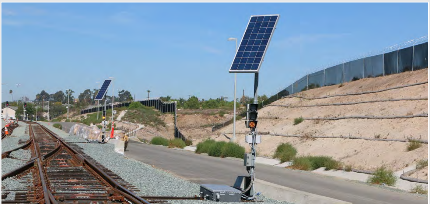
RailWorks completed a range of track improvements at the San Ysidro Freight Yard, including the installation of these two solar-powered GE switch machines.
