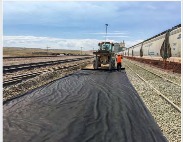
To prevent vegetation growth, crews installed 9,600 feet of geotextile fabric in the area between tracks in Solvay's rail yard. Once in place, the fabric is covered in ballast to keep it in place.
