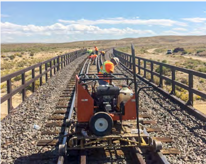
RailWorks installed guardrail on a 320-foot steel-girder, ballast-deck bridge on a spur that connects Solvay Chemicals in Green River, WY, with Union Pacific, the servicing railroad. The crew also changed out the cross ties on the bridge.
