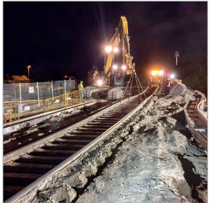
A track crew removed and reinstalled 90-foot track panels during the project.
