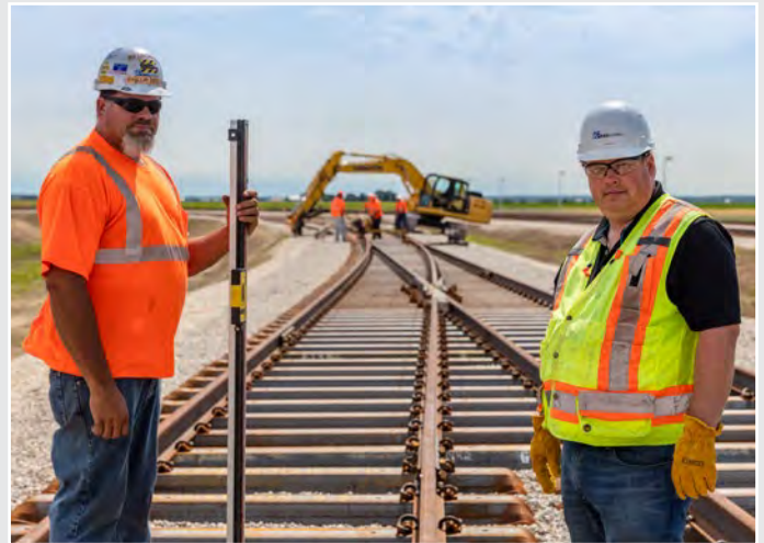
Project management on this job included labor and subcontractor management, handled by Phil DeClue (left), and contract and job-cost management, handled by Tim Wohlever (right), who also acted as liaison to the customer.
